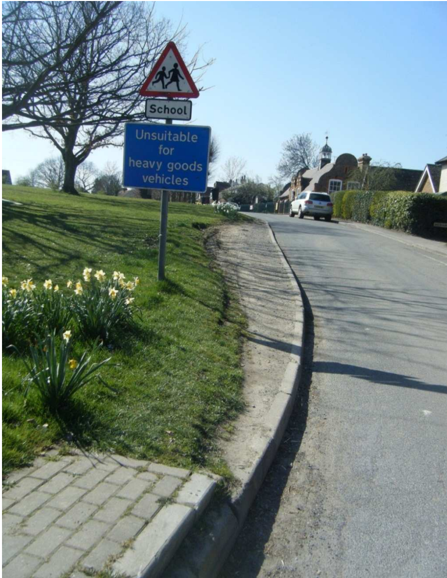
19. Damage to The Green by vehicles
